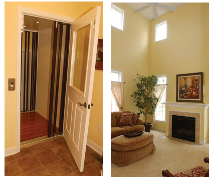
Above, the elevator makes four stops and comes with a hardwood floor (which matches what's in the house); a telephone; and a transparent accordion gate. At every level, the elevator is accessed through a door with leaded glass. The Parade house is 2,387 square feet and has 9-foot, first-floor ceilings.
